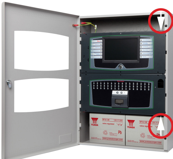
Figure 4-6 Opening the Fascia
