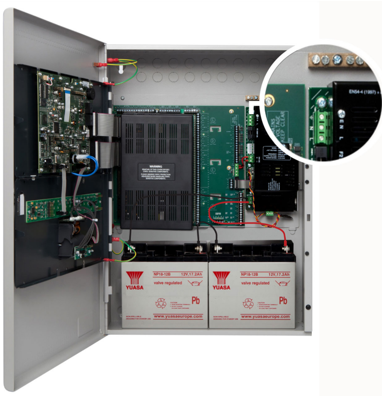
Figure 2-14 AC Power Connections of the 5.25 Amp Power Supply
